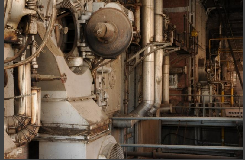
Fabra i Coats Power System
